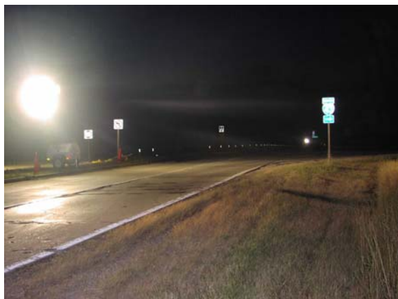
Figure 6-58 Portable Lighting (Photo courtesy of the Wisconsin DOT.)
