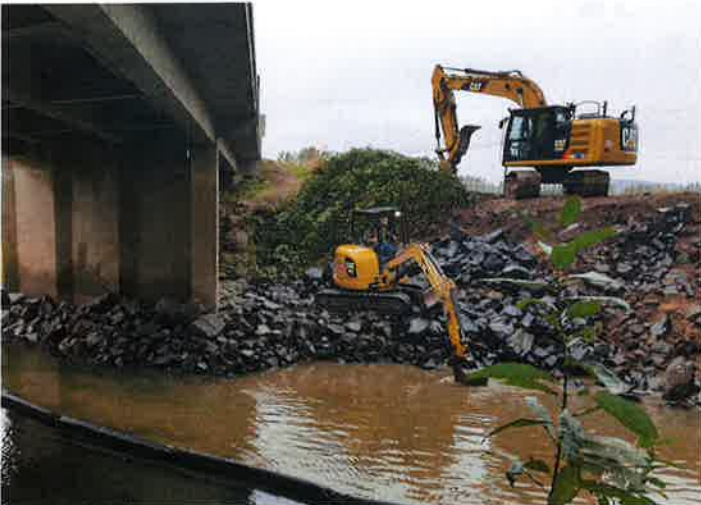
Erosion prevention project around a the base of a Polk County bridge.
