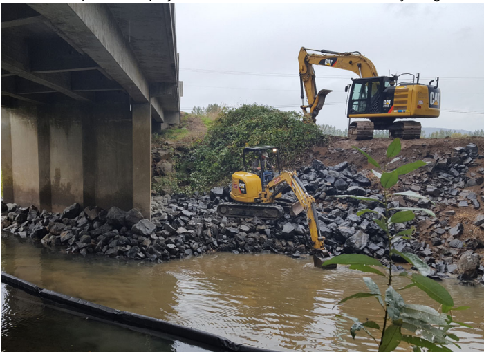
Erosion prevention project around a the base of a Polk County bridge.
